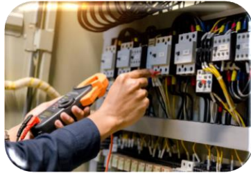
Electrical & Electronics / Telecom
